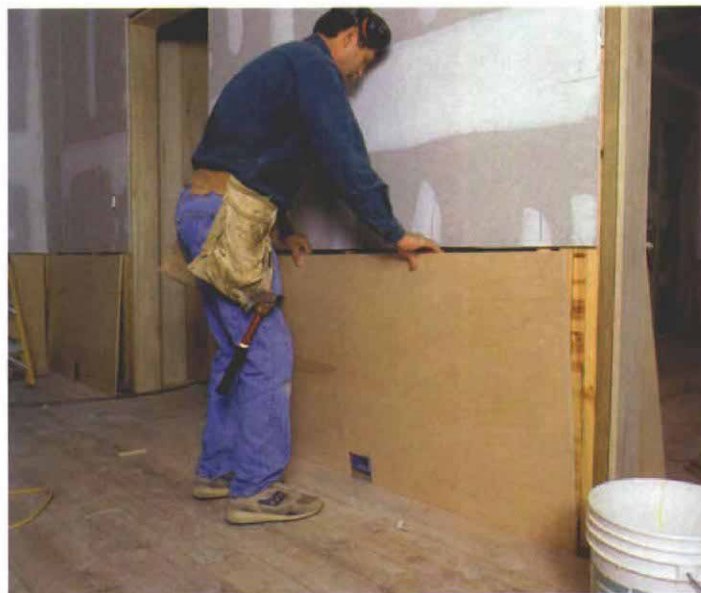
The plywood goes on first. A substrate of birch veneered plywood 1/2 in. thick, replaces the drywall from 31 in. down to the floor.
