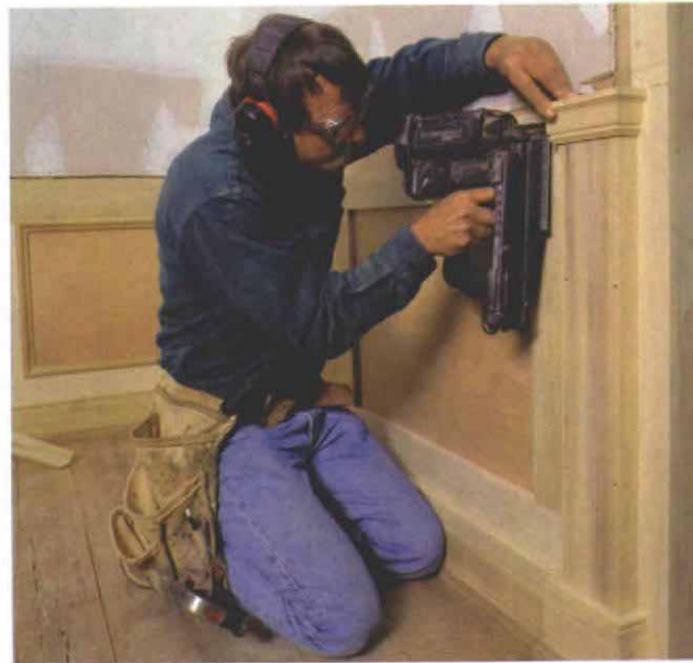
Moldings stop and start at the pilasters. At door openings, the pilaster and the flat subcasing provide a termination point for the chair rail, bed molding, and base and shoe.
